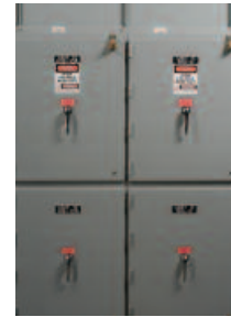
The arc resistant rear doors and plenum of a two-high design.
